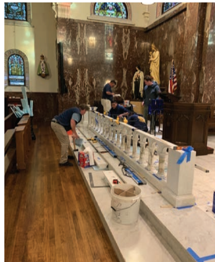
Installation of communion rails at St. Leo the Great Oratory was well underway last week. The communion rails had to be rebuilt after they were removed from the church when changes were made to the sacred liturgy at the Second Vatican Council.
