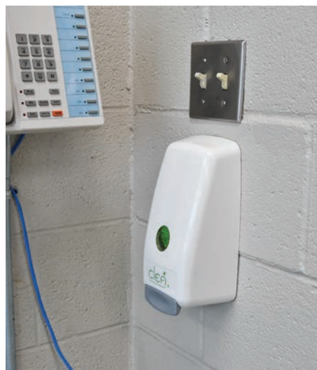
Hand sanitizers have been installed throughout Bishop Ready High School.
