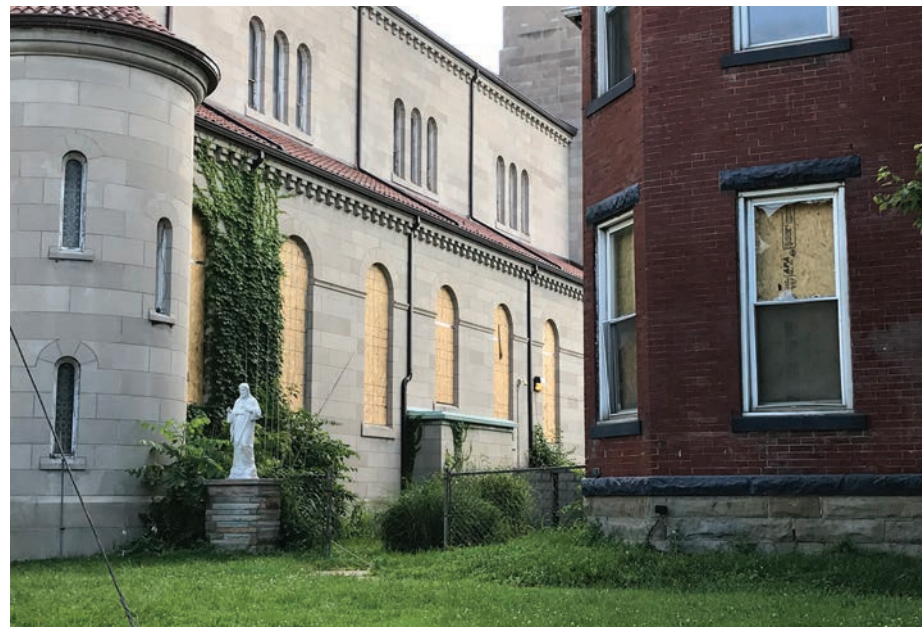
Columbus St. Dominic Church suffered damage as a result of a gas explosion which destroyed a nearby duplex on June 22. No one at the parish was injured.
