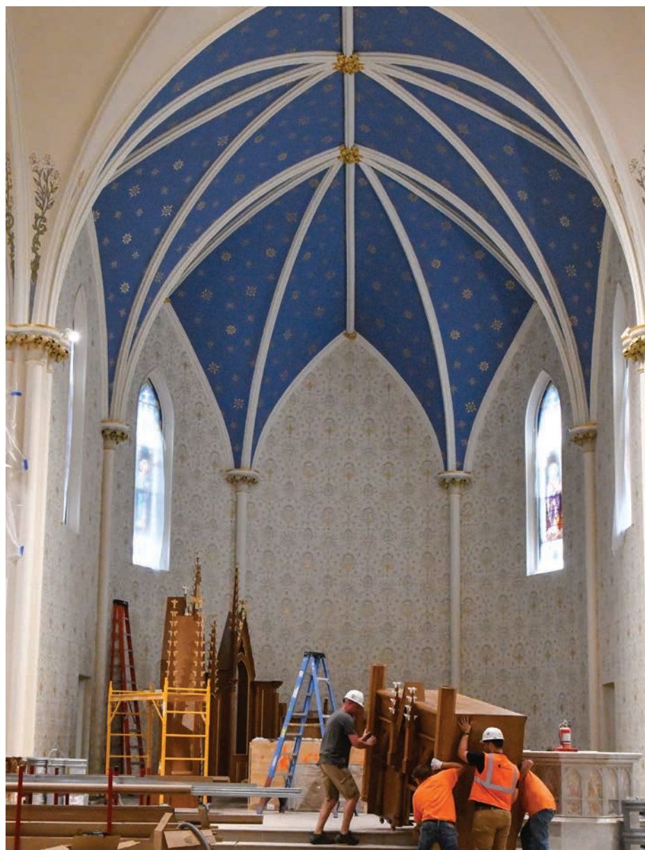
Workers move the reredos, which stands behind the altar, back into position at Lancaster St. Mary of the Assumption Church. The altar had been moved so the area behind it could be repainted during the church's remodeling. Two formerly blank panels of the reredos located above the altar will now include a depiction of Mary's Annunciation.
