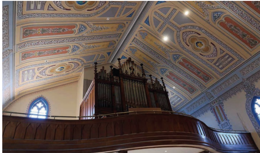
The church's organ stayed in place during the reconstruction and was enclosed in plywood while work was performed around it. An organ presentation will be part of an open house at the church at 2 p.m. Sunday, April 14, and will accompany a showing of the 1927 silent film classic "King of Kings" at 8 p.m. that night. Also shown are ceiling panels which depict some of the titles given to the Virgin Mary in the Litany of Loreto.
