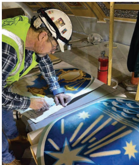
A worker from Martin Painting and Coating of Grove City prepares ceiling panels which match the originals. The new panels are canvases covered with digitally reproduced colors that look like paint.
