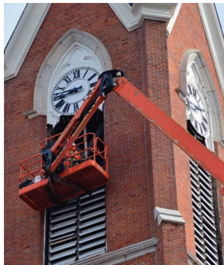
Workers repair the church’s bell tower. The bells were silent for 2 1/2 years as part of the renovation. The bell system is controlled by an electrical carillon system installed in 2012.
