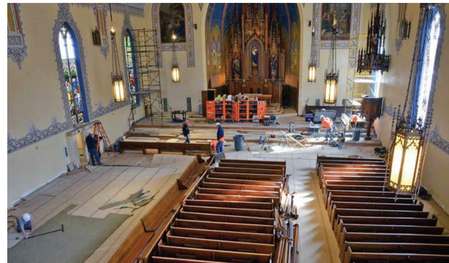
Workers were busy throughout the church once rebuilding got underway. It will look brighter because of enhanced lighting and because of the use of vibrant colors in painted scenes on the ceiling. The original paintings by liturgical artist Gerhard Lamers had been darkened by decades of dirt and smoke from candles. The pews shown are the originals from the 151-year-old building, the city’s third-oldest Catholic church.
