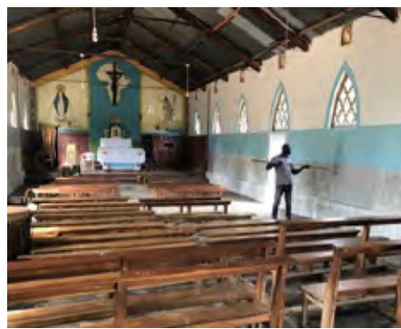
A man paints the inside of a church in Uganda. Photo courtesy Diocese of Arua
