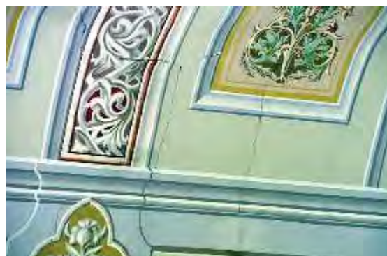
Cracks in the ceiling of Columbus St. Mary, Mother of God Church, caused by a lightning strike on Sunday, Aug. 28.
