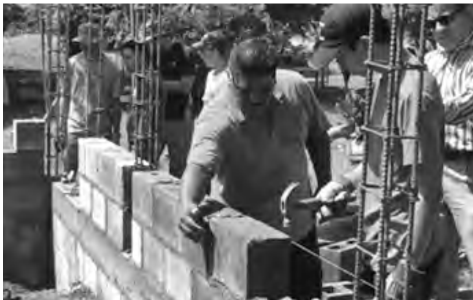
David Suh takes instructions from a foreman while building a new classroom in Esquintla, Guatemala.
