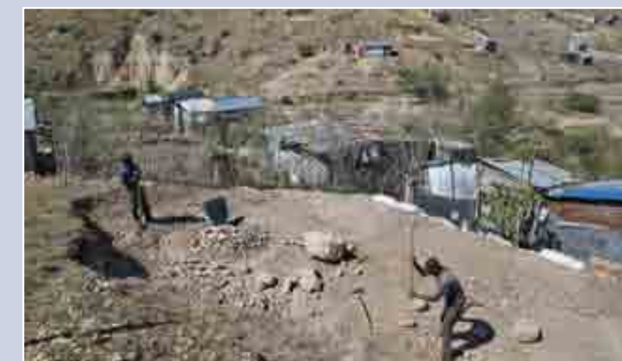
Men work on leveling ground to build a new home in Cnaan, a community on the outskirts of Port-au-Prince, Haiti, on Feb. 17. Cnaan, which has an estimated 250,000 inhabitants, emerged soon after the 2010 earthquake, when the government said people could relocate there. CNS photo/Bob Roller
