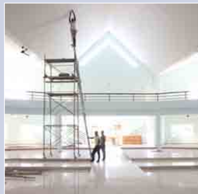
Men work on the partially completed multipurpose center for the Cathedral of St. James and St. Philip in Jacmel, Haiti, on Feb. 12. The cathedral was left unusable by the January 2010 earthquake and is being rebuilt by Partnership for Church Reconstruction in Haiti. The center will host Masses until a new cathedral is built.
