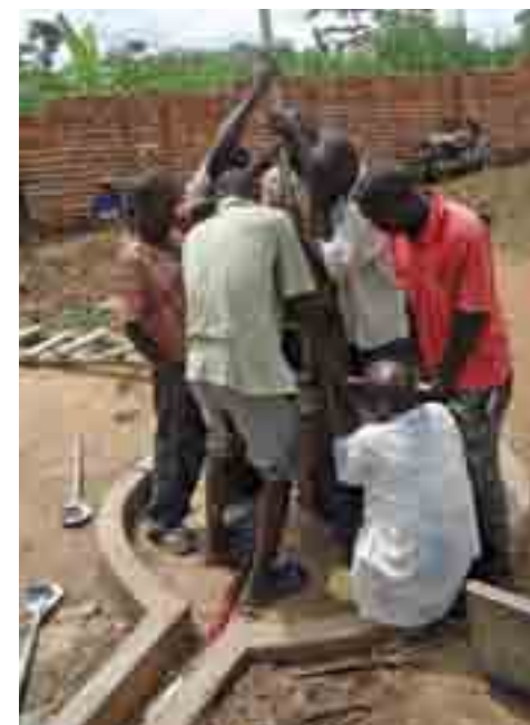
Men of the community around the Kagoma Orphanage in west Uganda repair its well. Money to pay for the work was raised by Father Bernard Bitekerezo during a visit in April to central Ohio.
