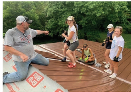
Chuck Schafhausen explains roofing to Appalachian Project volunteers (from left) Emilee Zoog, Keegan McKnight, Evie Campbell and Grace Eisenstein.
