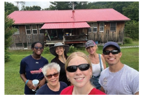
The roofing team at the Anawim house includes (from row from left) Rita Frye, Ingrid Bedell, Thai Trinh; (back row from left) Kaitlyn Acquah, Eva Padilla Barroso and Lisa Horn.
