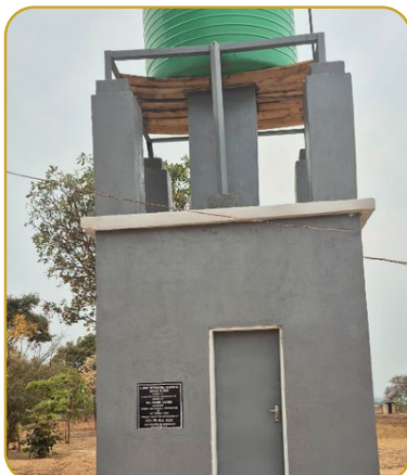
The 5,000-litre tank above the new borehole
