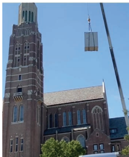
One of two 15-ton condensing units for the new air conditioning system in the Pontifical College Josephinum's St. Turibius Chapel is lifted by crane before being hoisted through the balcony of the college's bell tower. Photo courtesy Pontifical College Josephinum
