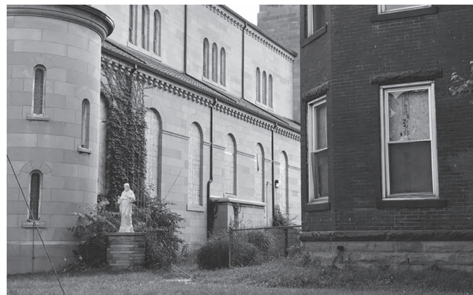
Stained glass and rectory windows at Columbus St. Dominic Church sustained extensive damage from a nearby gas explosion on June 22. CT photo/Doug Bean
