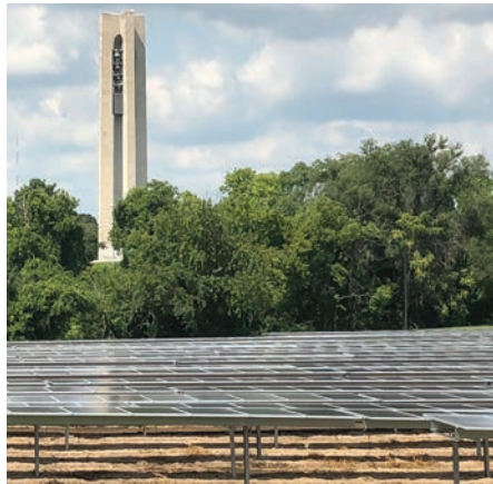
Solar array at Dayton. Photo courtesy UD
