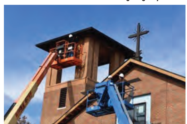
Efforts to rebuild the church began shortly after the fire. Workers are shown at the bell tower during some of the final stages of construction. A new church was dedicated on Thanksgiving 2015. Photos courtesy Sacred Hearts Church
