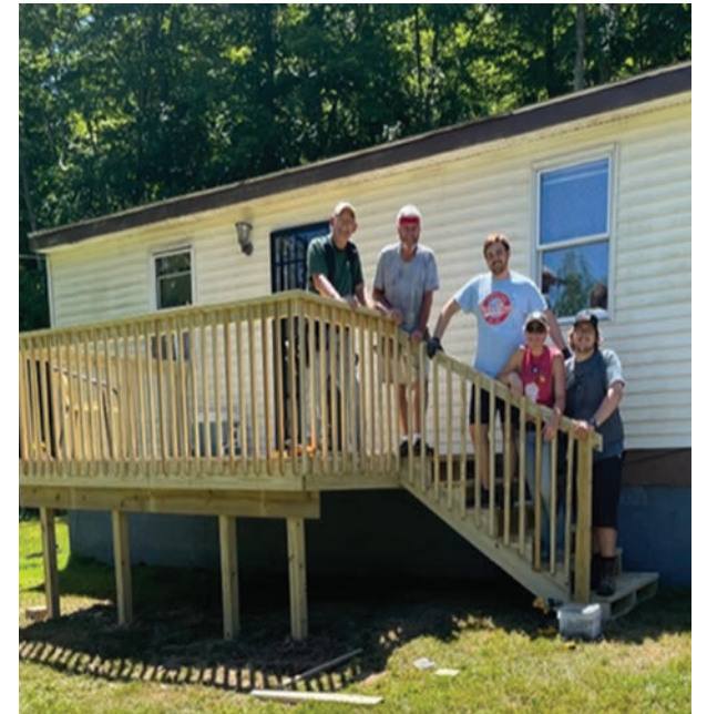
A new deck and steps were provided for a home in western Scioto County by volunteers (from left) Jim Schafhausen, Jeff Gardner, Hudson Ozello, Madison Schafhausen and Corey Claprood. Photo courtesy Anne Jupinko
